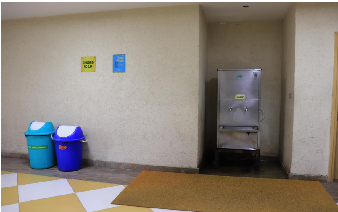
Picture 2: Water cooler installed across the university campus
